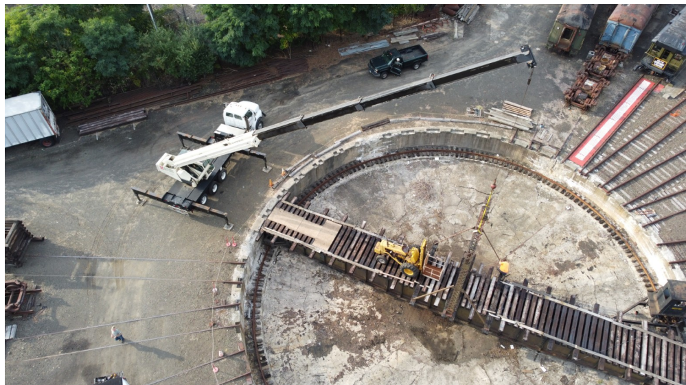
Left: Mariano Bros' crane is positioned to carefully remove the 104-year old structure.
