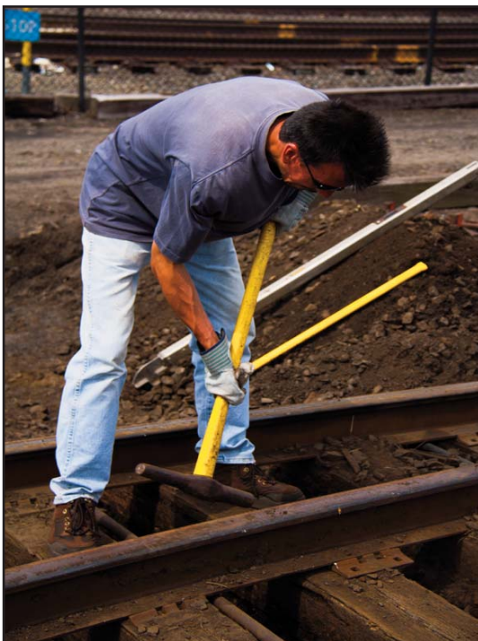
Left: After digging out a majority of the last two remaining switch timbers on the east end, Mike Madyda uses the spike maul to knock out the tie plates to prepare them for removal. Right and bottom right: Justin scrapes away dirt and ballast using the backhoe at the north end of the timbers to make removal easier.
