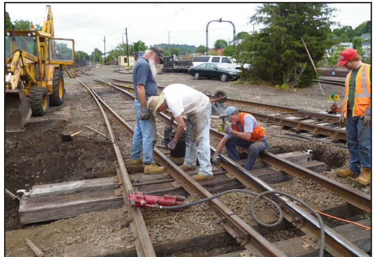
After the switch timber has been jacked up, Jeff drills holes to receive the rail spikes while Don holds the tie plate down with his foot. Behind Jeff, Jim starts the spikes into the holes.
