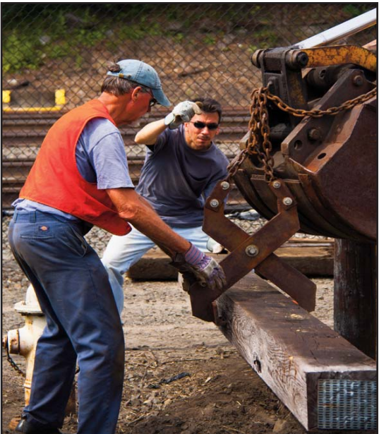
Left: Mike gives the backhoe operator (Justin) directions where to place the new switch timber as Jim steadies it. Photo courtesy of Philip Beard. Right: New switch timbers placed under the rails ready to be lifted and secured to the rails.
