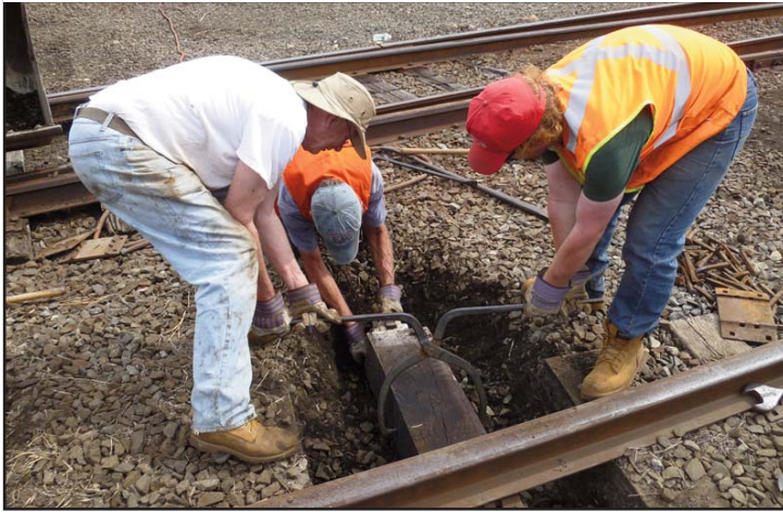
Jeff and Philip lifting one end of the timber so Jim can get the rail jack under it.
