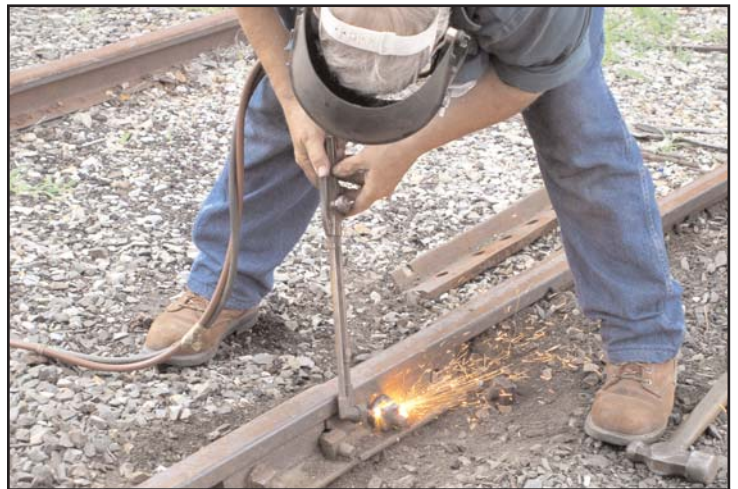
Bob Pitcher torches a bolt out of a rail joint bar. The joint bar was broken and needed replacement. Bob found this a good opportunity to teach some other volunteers how to use a torch for cutting.
